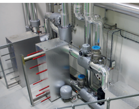
Supply circuit at 90°C – a Viegand Maagøe A/S solution.
