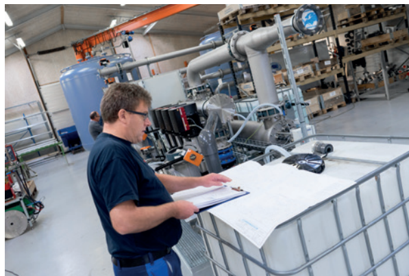
After production and pre-assembly, the water treatment solution and the documentation was inspected by all relevant parties; manufacturer, customer, installation company, and supervisor.
