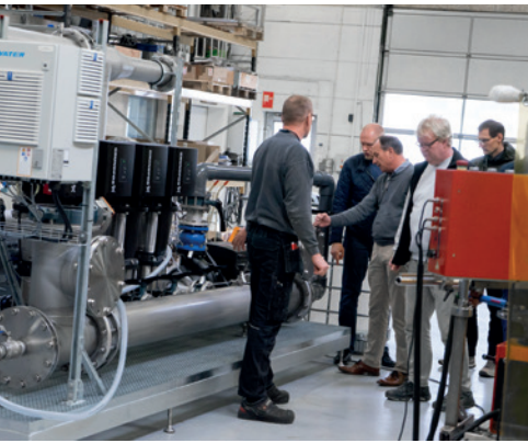
Inspection of plug-and-play frame-mounted unit with booster pumps and UV disinfection system.
