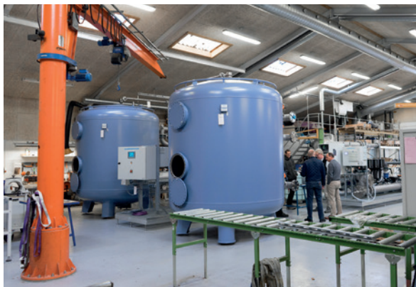
Two pressure filter type TFB from EUROWATER. Between the filters is a pre-assembled skid with PLC control cabinet as well as equipment for backwash and UV system.
