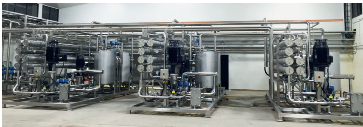
Reverse Osmosis plant from GEA.
