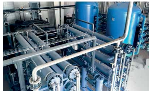
Complete water treatment solution based on pre-engineered EUROWATER units for RUD, Ukraine.
